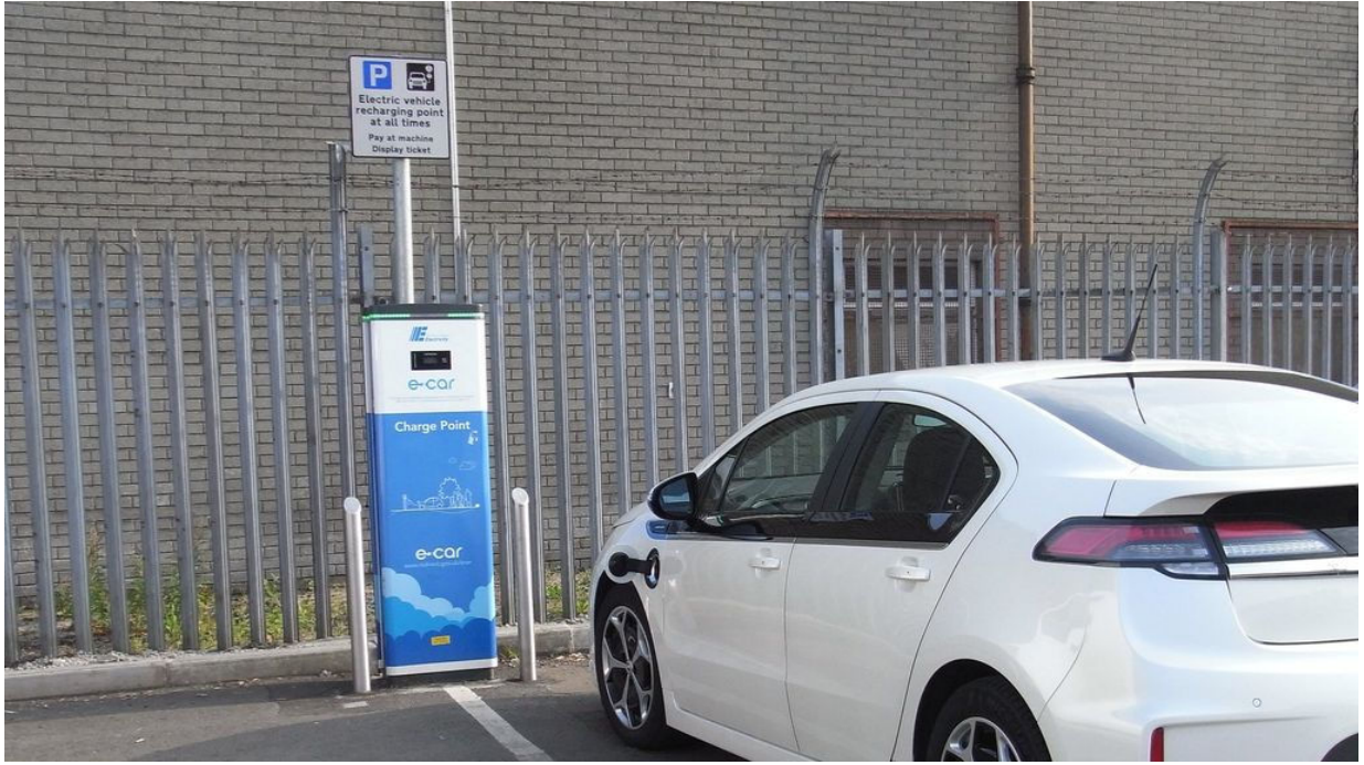
Figure 4 - E-Car charge point
